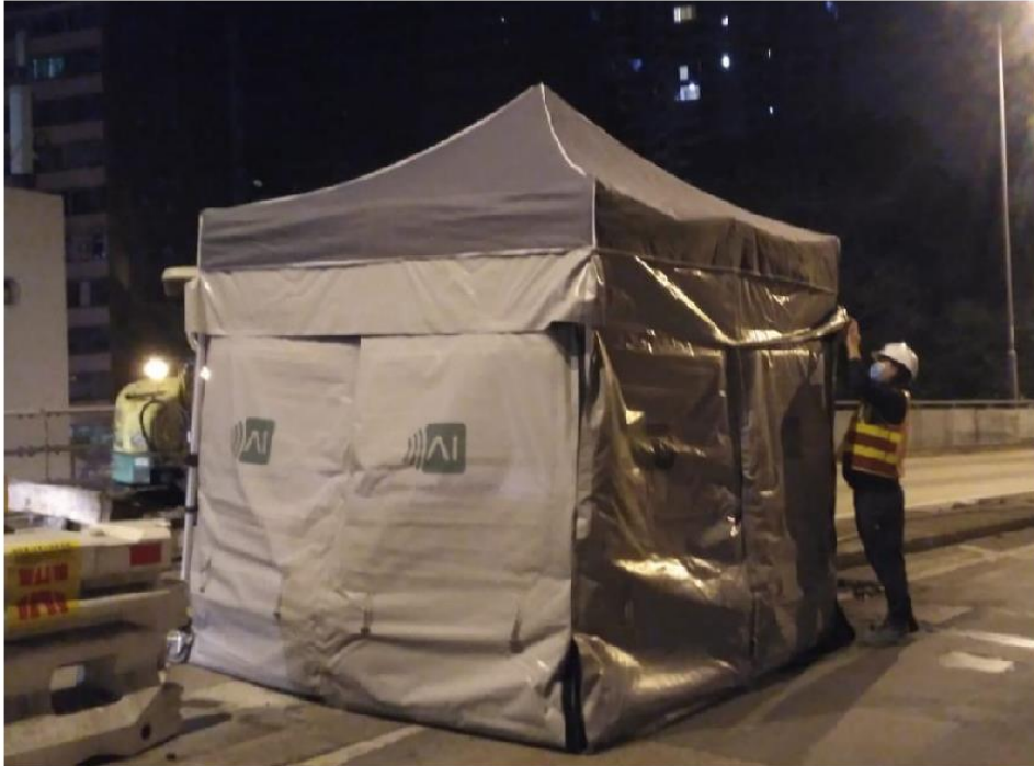
Figure A: Movable Acoustic Enclosure (SilentCUBE) that the Contractor used at the work site on 20 January 2022
